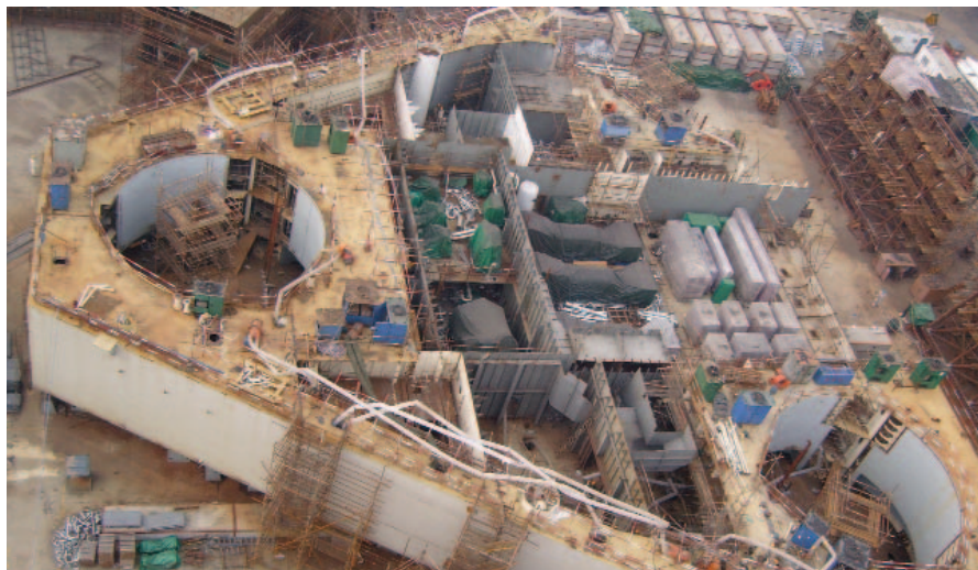
Figure 2. Construction of the first ESV combination rig/vessel well intervention unit continues at Cosco (Nantong) Shipyards.
